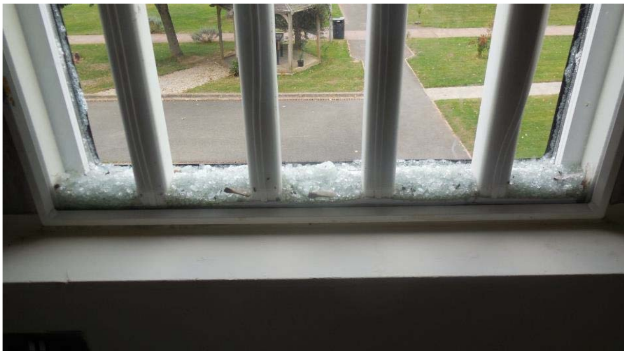
Below: Broken window on LB 8.
