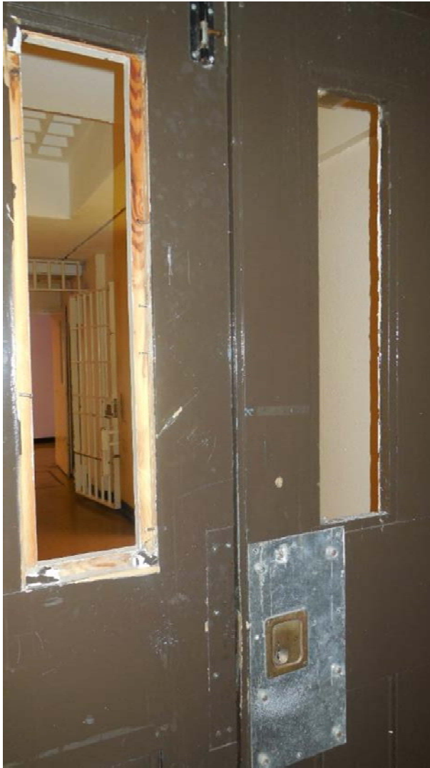
Left: Missing window in door, LB I.
