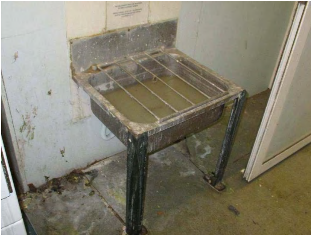
Photograph 7. B wing laundry blocked sluice with dirty floor
