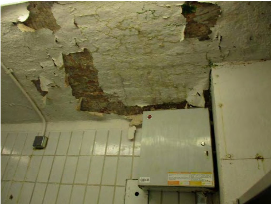
Photograph 6. A laundry leak onto an electrical box
