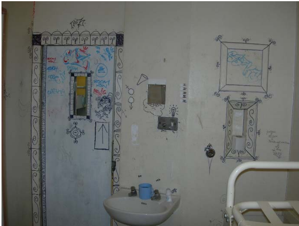
Extensive graffiti in first night cell on house block 4
